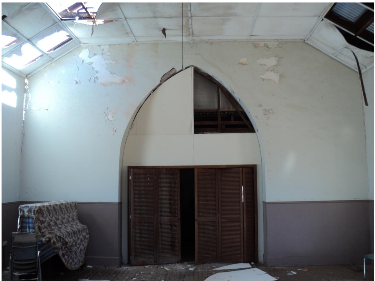
Cyclone Seroja damage 2021
