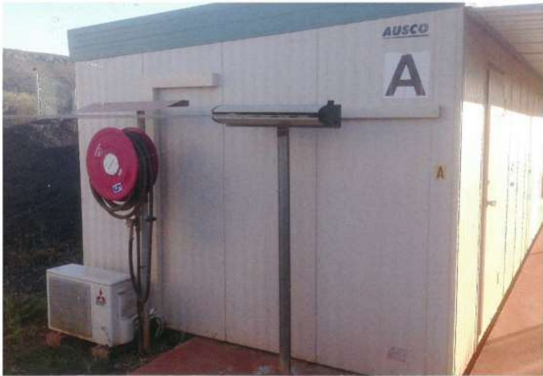
Above: View of side of relocated building (existing hose reel would be removed) this is proposed to be the western elevation on Lot 18
