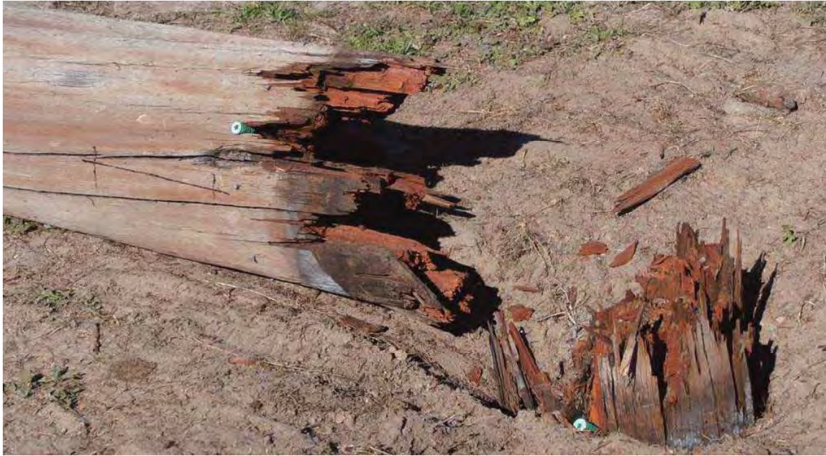
Figure 6 - Complete failure of Jarrah wood pole due to decay/rot at ground line
