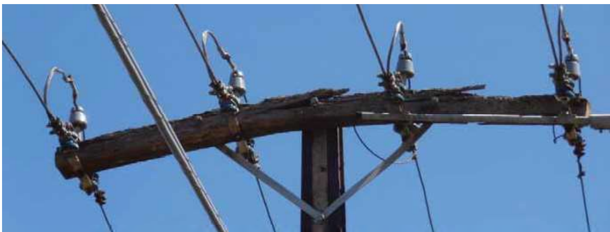
Figure 8 – A badly split low voltage crossarm
