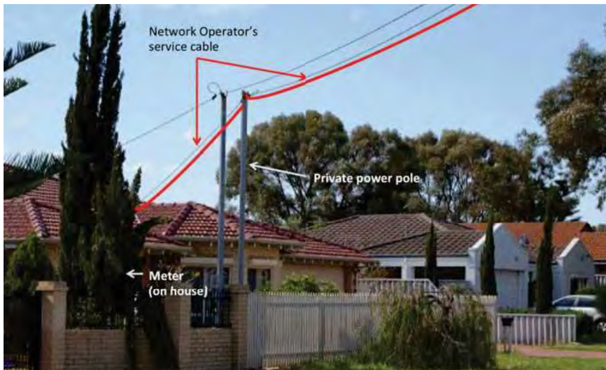
Figure 2 - Typical urban residential private poles supporting network operator's service cables
