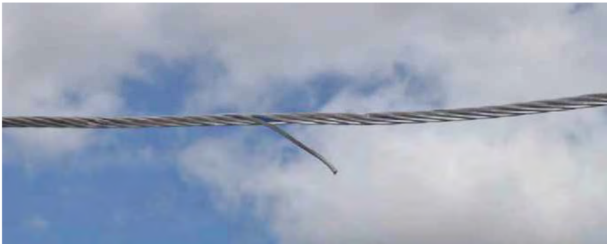
Figure 11 - Broken conductor strand clearly visible
