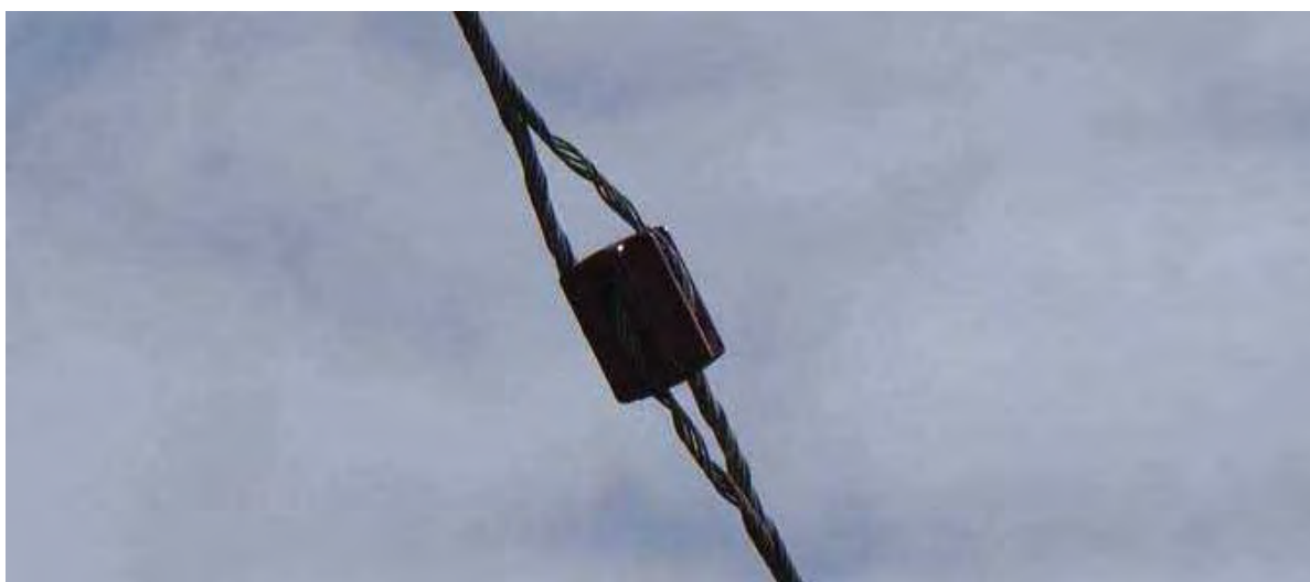
Figure 10 - Stay insulator correctly installed and in good condition
