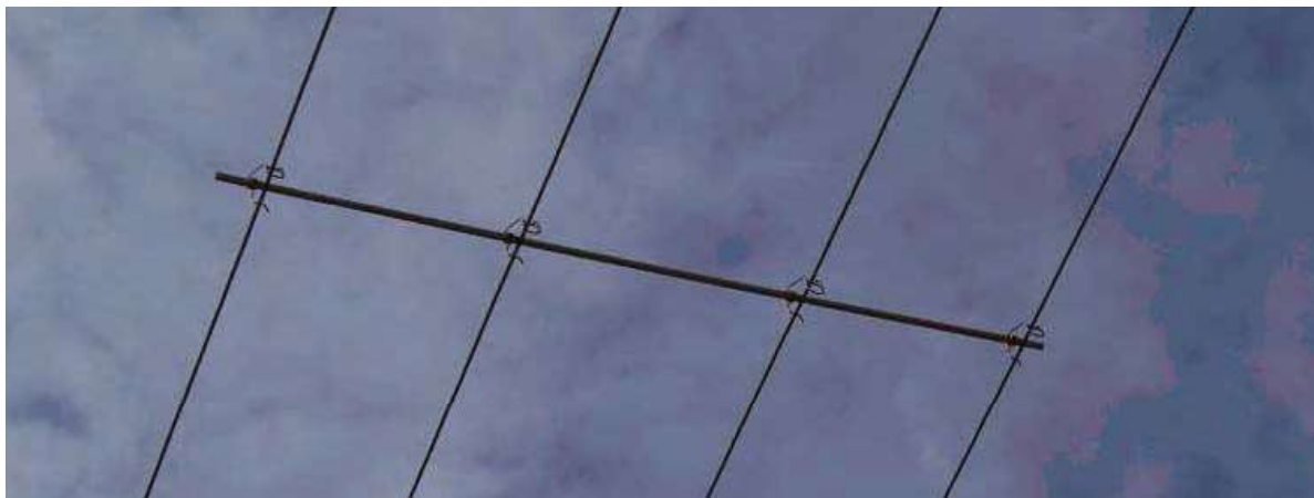
Figure 9 - Low voltage spreader in good condition
